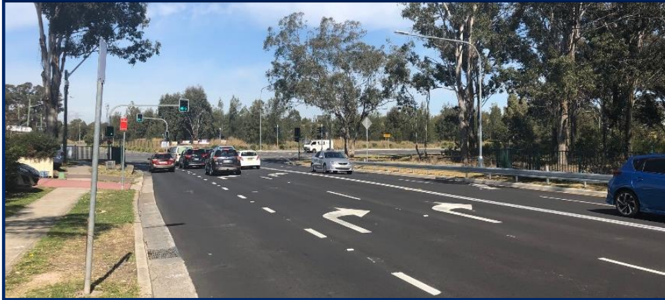
Additional right turn lane from Hoxton Park Road onto Whitford Road, Hinchinbrook
