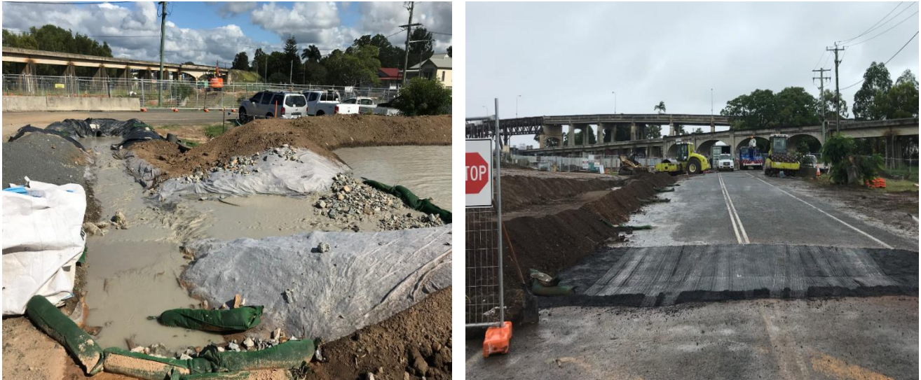
Figure 12 Controls installed to manage piling water during air lifts and pile pours in Grafton (left) and additional controls and drains installed along Kent Street, Grafton to manage potential dirty water run off (right)
