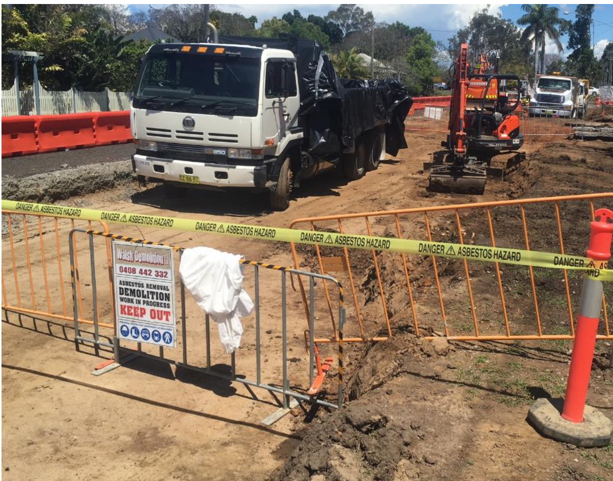
Figure 4 Removal of bonded asbestos into a lined truck to be taken to Grafton landfill
