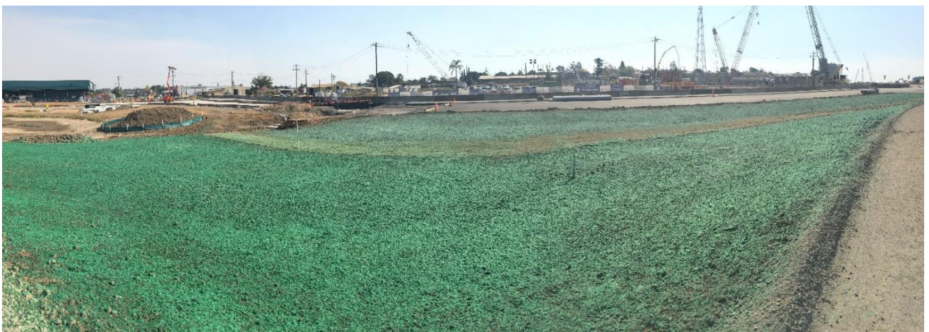
Figure 9 Hydromulch and coir mesh application on disturbed ground diverting water into Fill 2 Basin.
