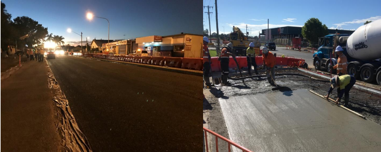
Figure 3 night works along Pound Street (left) and new footpath construction on Iolanthe Street, South Grafton (right)
