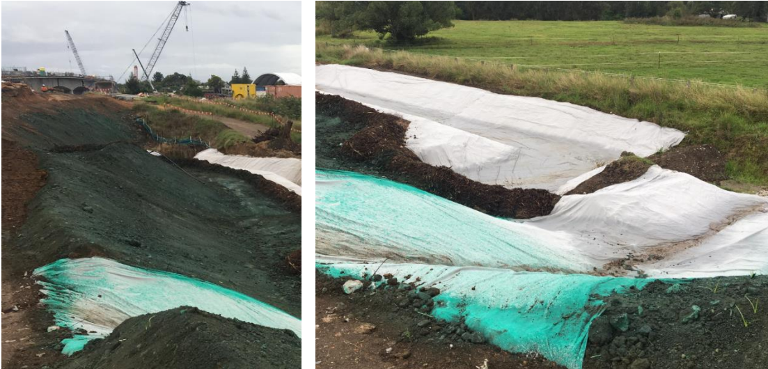
Figure 10 Polymer application to an exposed batter on fill 1 (left) and an example of how clean and dirty water separation is being maintained (right).
