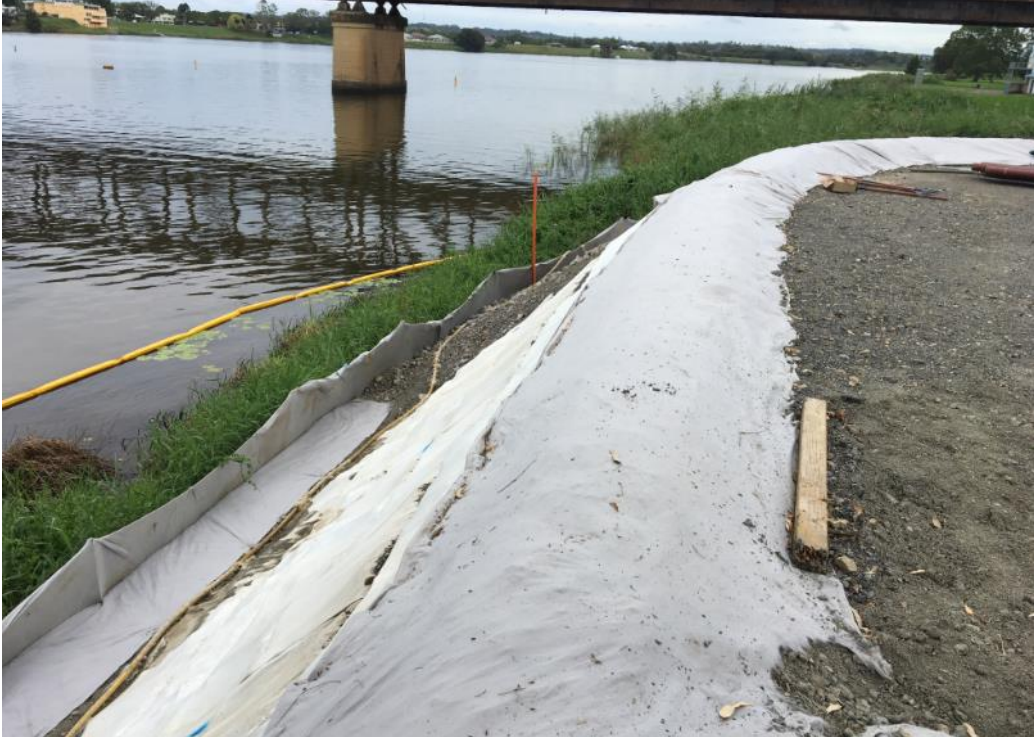
Figure 5 Northern crane pad on the banks of the Clarence River, photo is looking east
