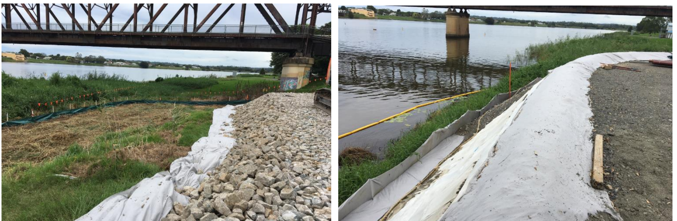
Figure 11 Perimeter controls installed ahead of the northern levee pipe jacking works (left) and the northern crane pad extension (right)
