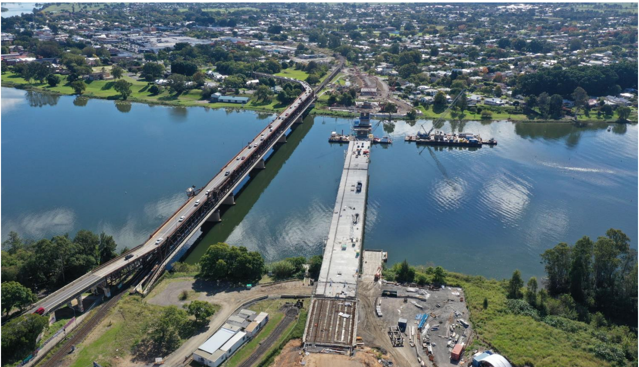
Figure 6 Significant progress has been made on the new Grafton Bridge during the reporting period
