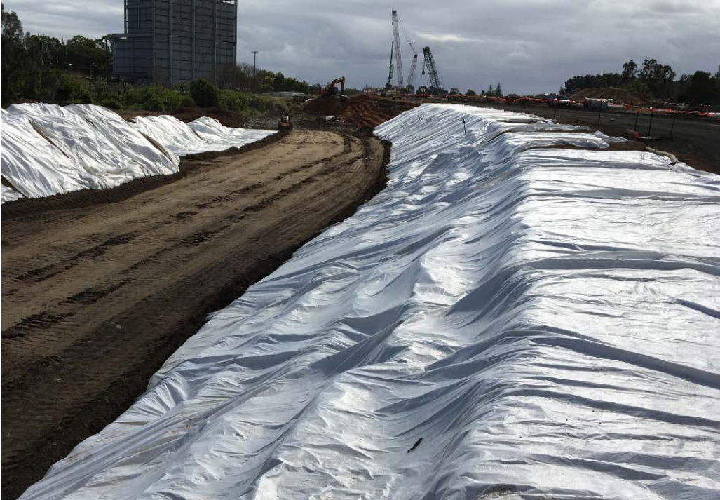
Figure 4 Asbestos contaminated material being encapsulated in a batter widening for future infrastructure
