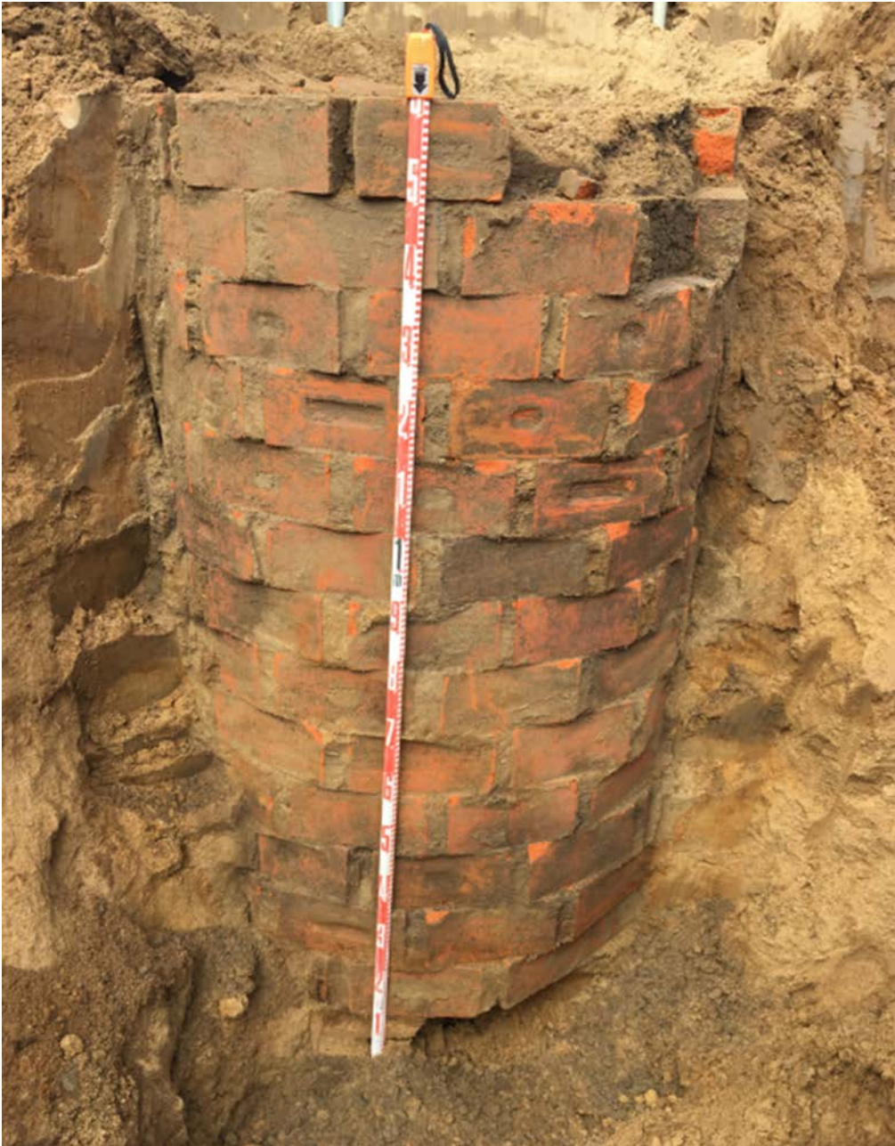
Figure 12 A cistern was located whilst excavating to install the pump station gravity main in Grafton
