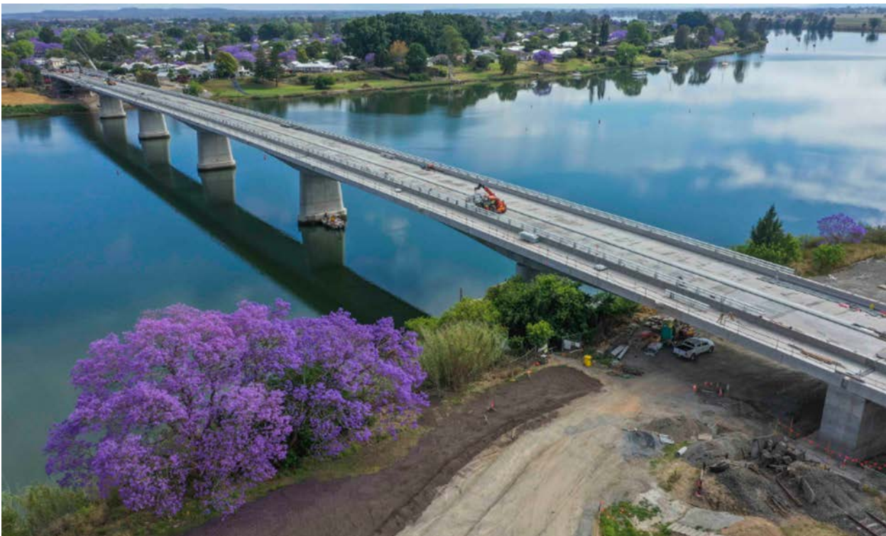
Figure 6 Significant progress has been made on the new Grafton Bridge during the reporting period
