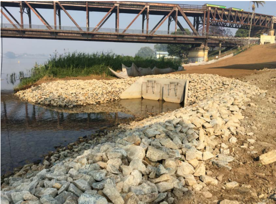
Figure 1 Outfall structure of the northern pump station
