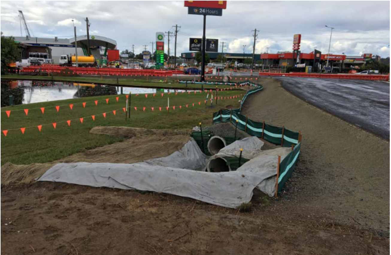
Figure 10 best practice erosion and sediment controls installed for temporary pavement and drainage works
