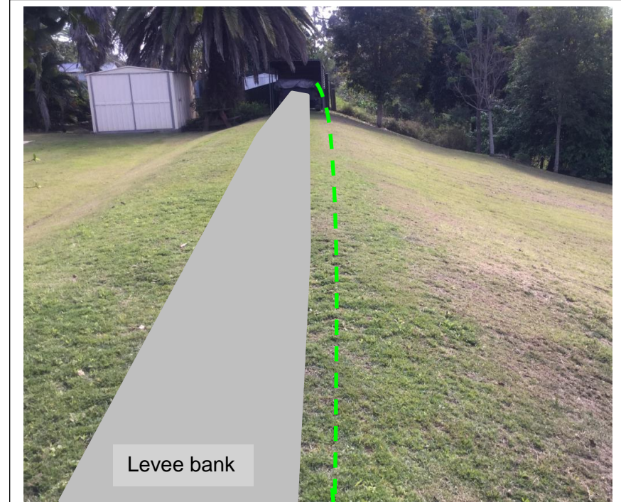
Example scenario 3: Embankment works controlled with a sediment fence on the downstream side, installed prior to works starting
