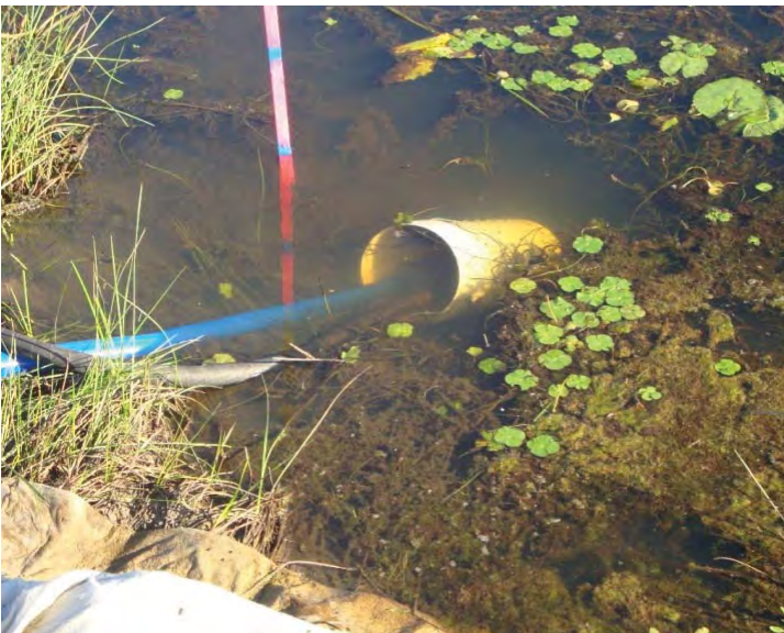
Figure 2. Consideration should always be given to measures to prevent pumped inlets from falling into sediment zones at the bottom of basins. In this example an anchored bucket was seen to be effective.
