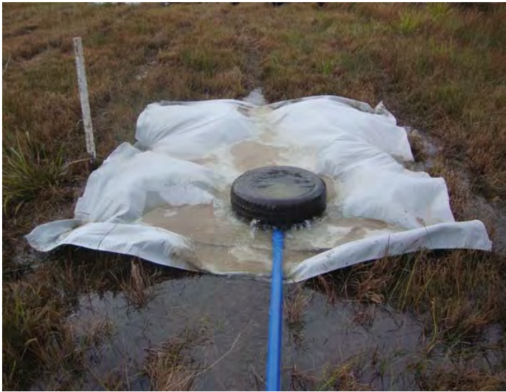
Figure 3. Informal use of bunding and geotextile was assessed as a suitable outlet treatment for scour protection in this example. The use of a tyre provided both energy dissipation for the discharge flow and anchorage for the discharge pipe.
