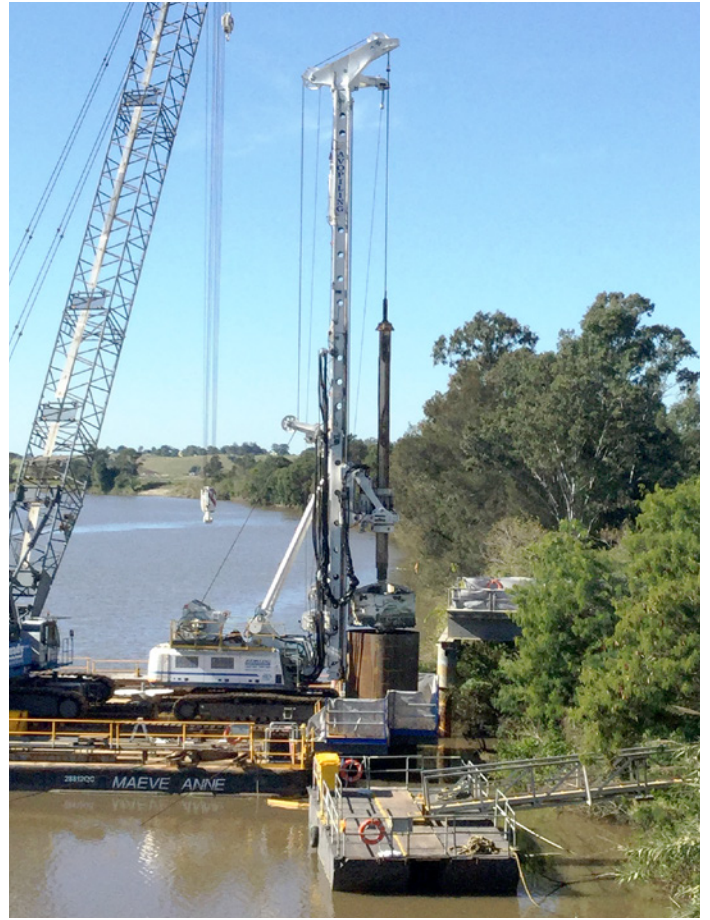
The BG40 piling rig boring the first pile in the Clarence River
