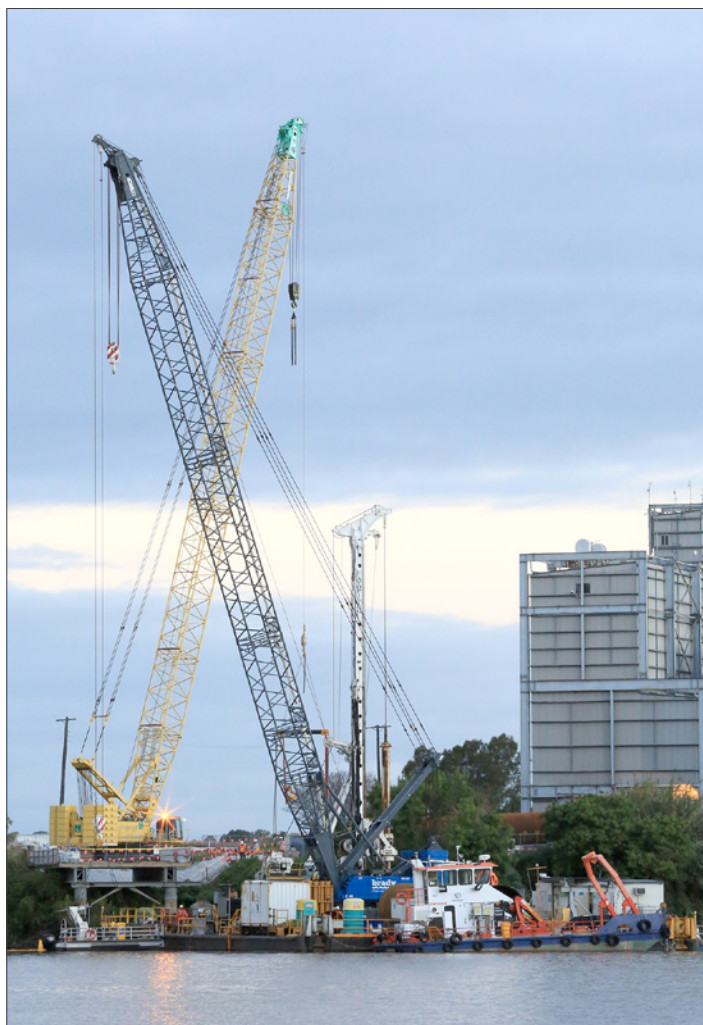
The barge, cranes and piling rig, which will be used for river piling
