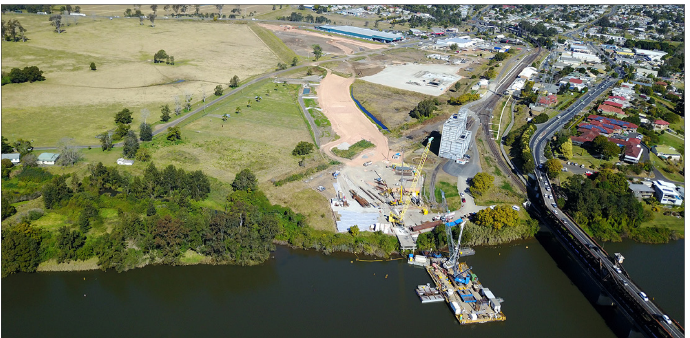
Aerial photo looking south towards land and marine piling, soft soil work and pre-cast facility.
