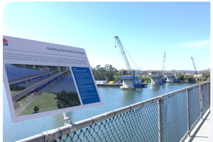
Signage on the existing bridge explaining the build of the new bridge
