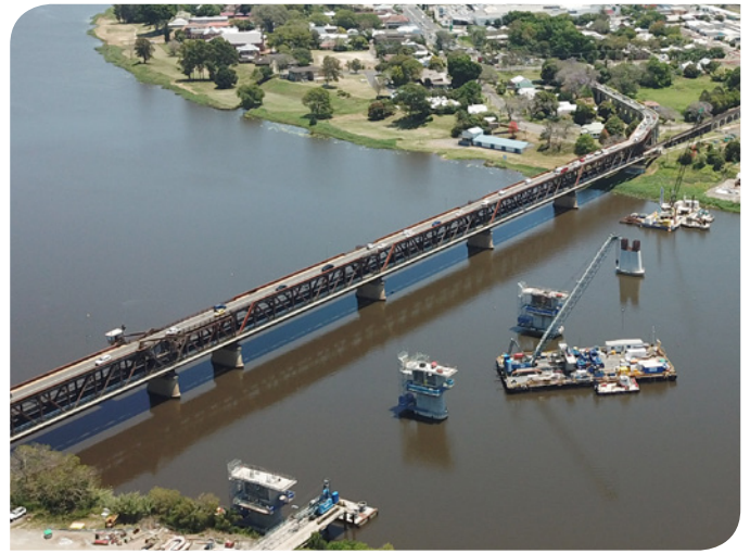
The new Grafton Bridge under construction looking from south to north (November 2018)
