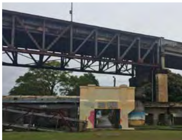
Fig. 4-44: View of the existing bridge and railway viaduct on North Grafton side.
