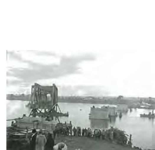
Fig. 8-33: Floating the first pier into position at South Grafton on Monday 26 May, 1930 (CRHS). Source: Fruits of Federation, The Grafton-Brisbane Uniform Gauge Railway and the Clarence River Bridge, Robert Lee, page 67.
