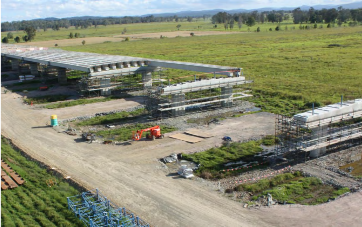
Figure 50: Example of prestressed beam-and-slab (Super-T girders) construction method – Kempsey (New South Wales)
