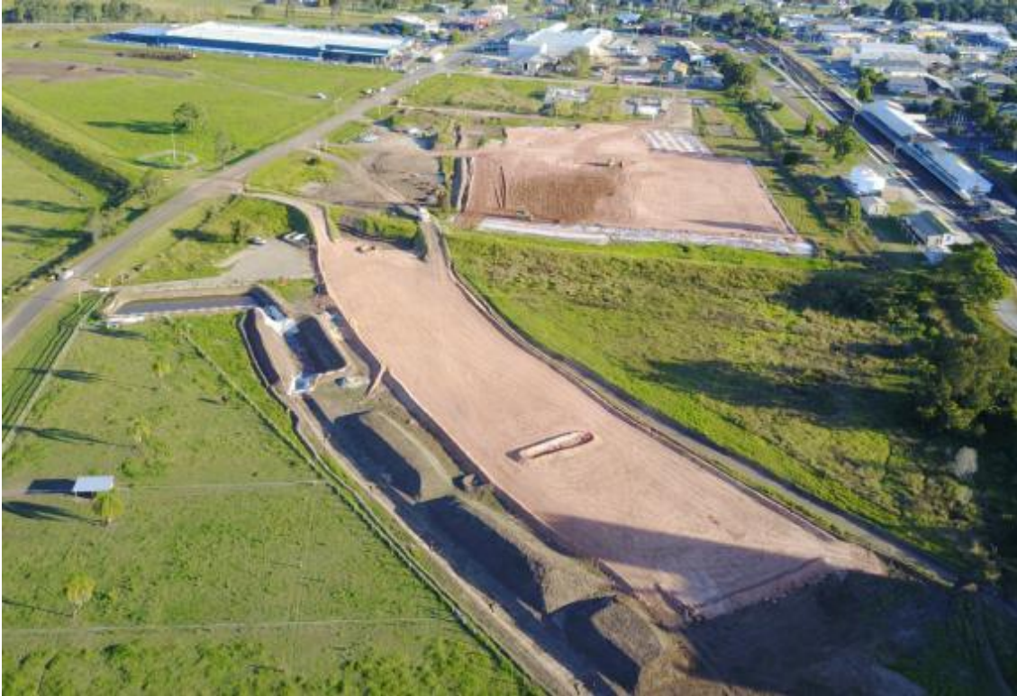
Figure 4 Fill 1 (foreground) and casting yard (background) work progress demonstrating ESC and sediment basins. Site runoff is being diverted away from the Clarence River at Fill 1 and directed towards the sediment basins and erosion/ sediment controls beside the fill.
