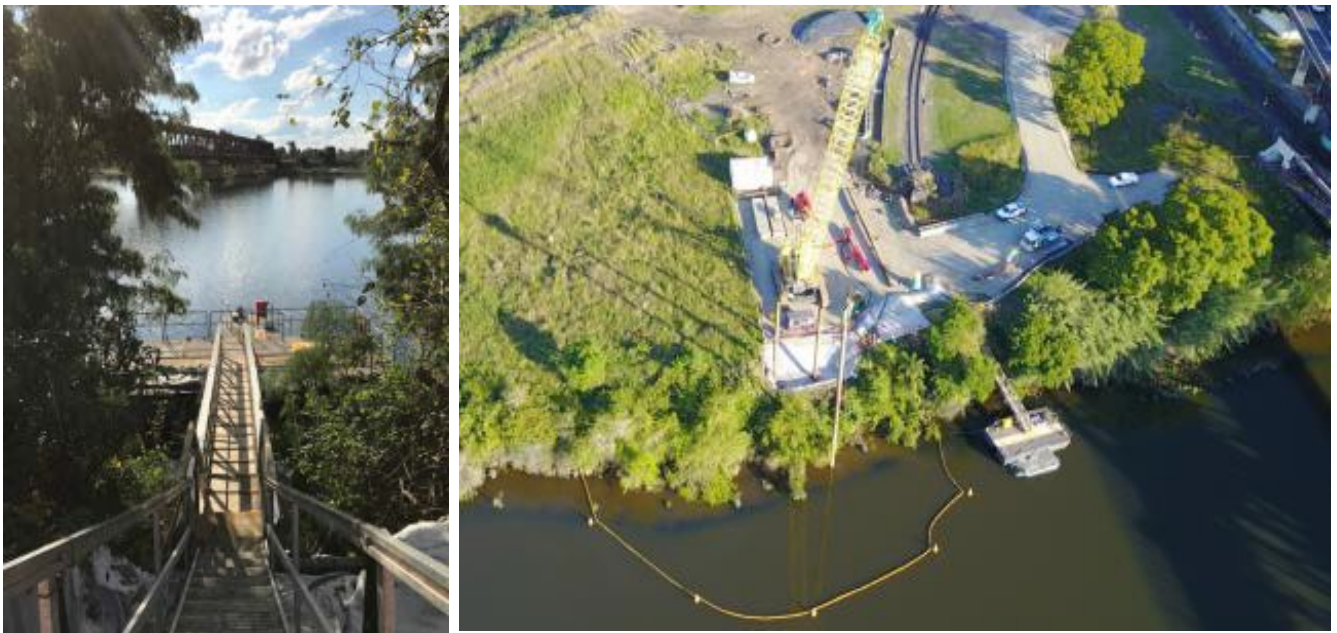
Figure 7 (a) Temporary walkway and (b) early construction of the marine works jetty
