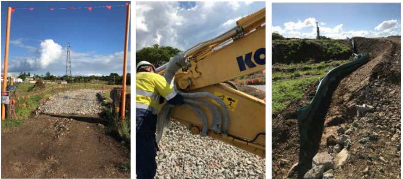
Figure 9 (a) Clean rock access tracks to prevent mud tracking onto local roads, (b) sheathing of excavator hose lines when working around waterways for easy identification and containment of leaks and/or breaks, (c) mulch bund reinforced with a sediment fence
