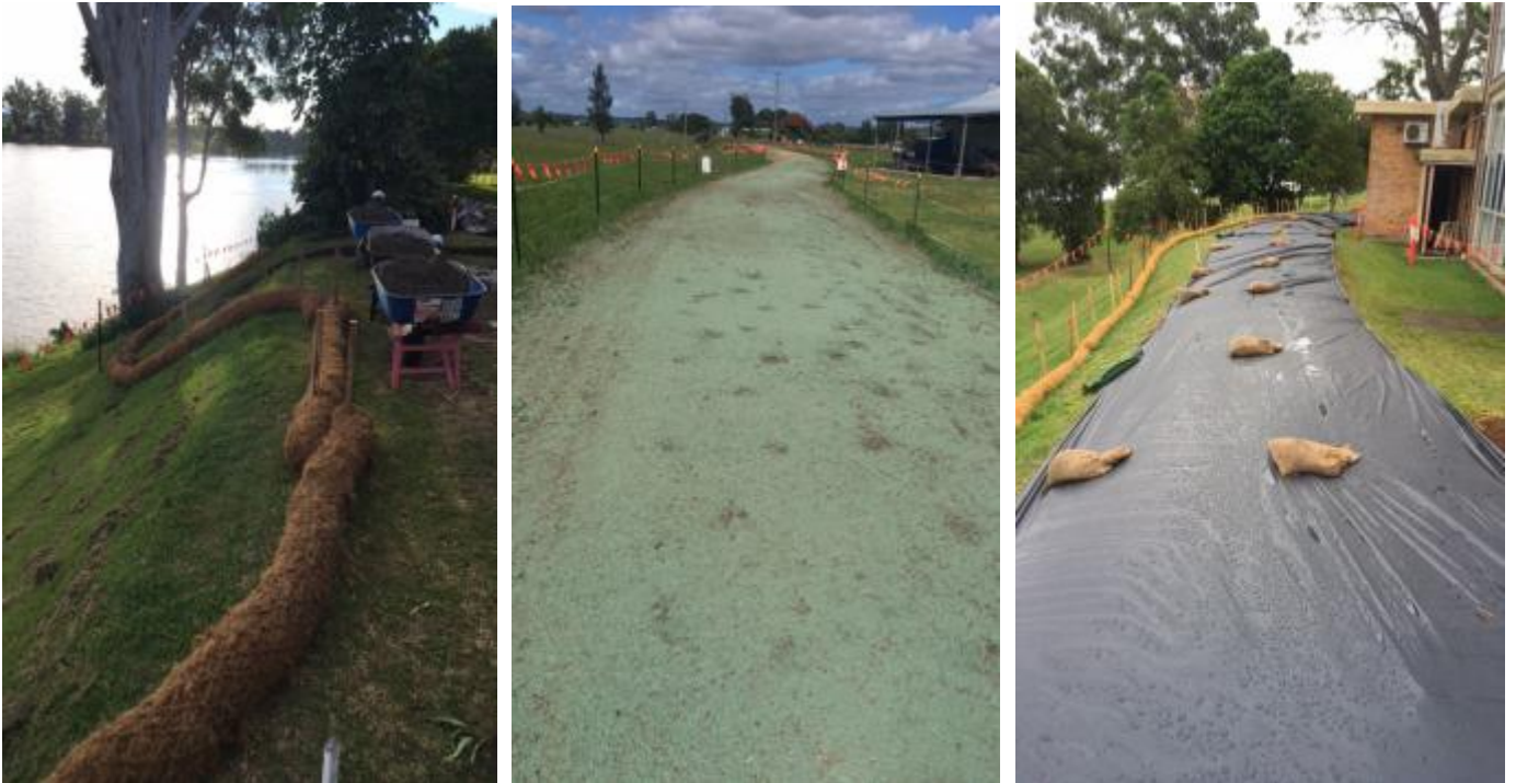
Figure 1 Levee works highlighting the focus on narrow works corridors and the range of alternative erosion and sediment controls used for these works
