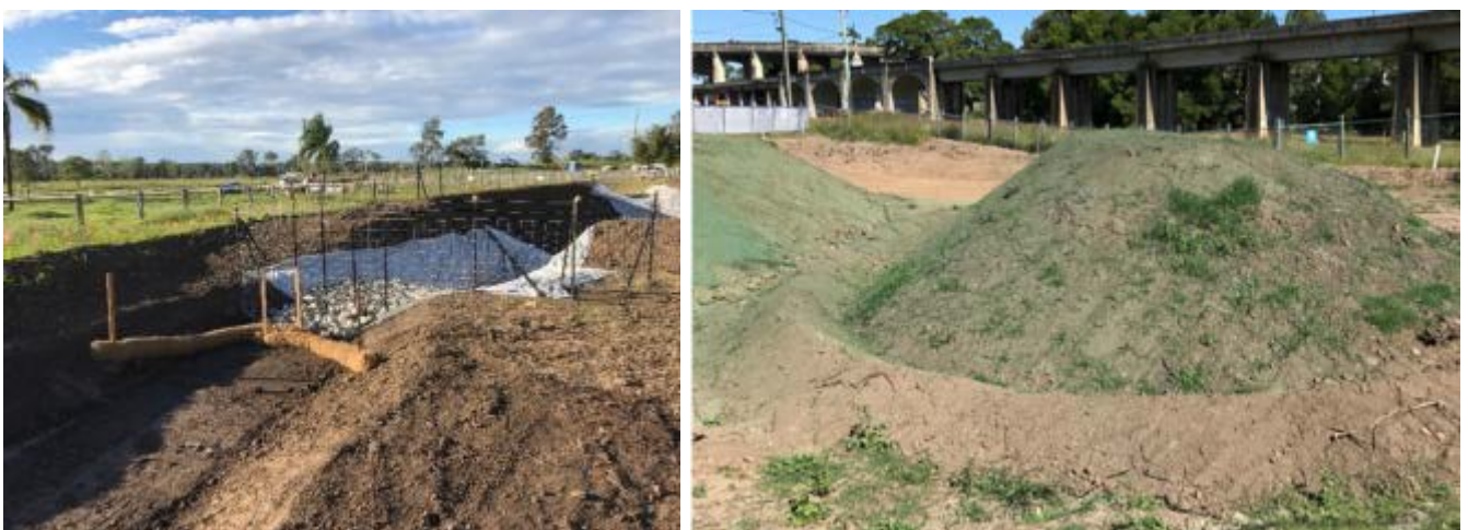
Figure 6 (a) Site dirty water drain and coarse sediment trap, (b) polymer application on stockpiles
