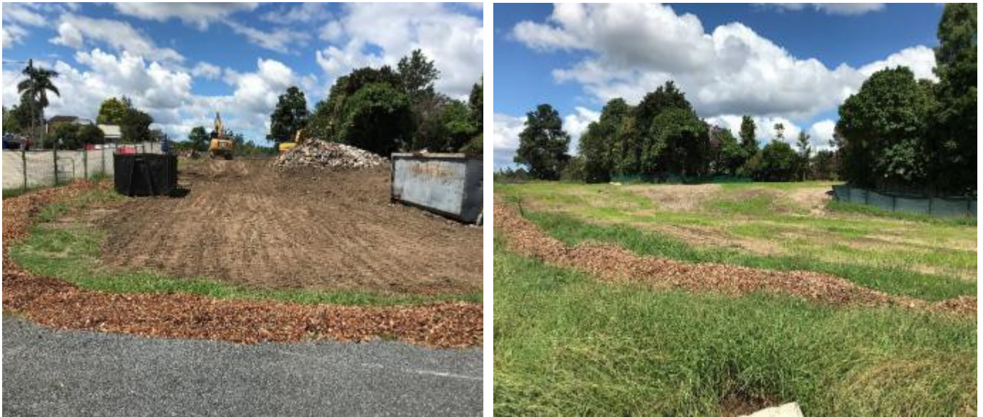
Figure 2 Site rehabilitation following demolition works, note mulch controls and good cover crop growth.
