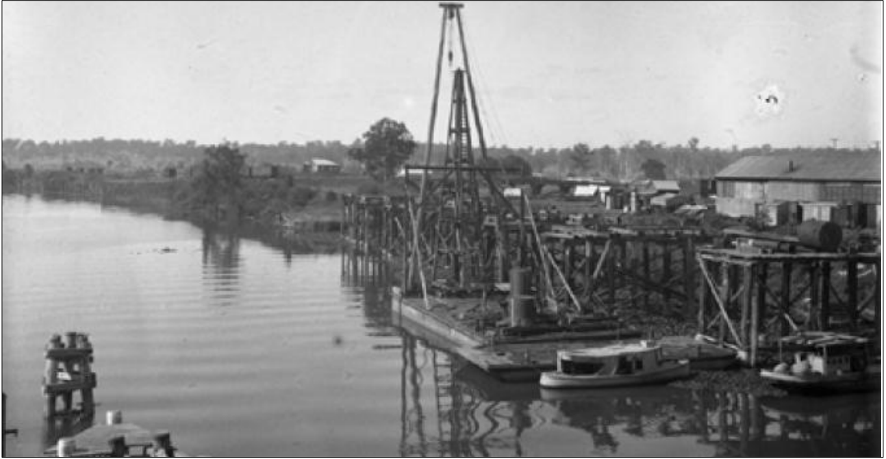
Plate 14 Onshore facilities and wharves photographed during construction of the Grafton Bridge at South Grafton c.1930. View is eastward from the bridge over the former wharf reserve toward the Railway Precinct terminus and project area (Source: Engineering Heritage Australia report: Grafton to Brisbane National Railway Link 2009:26)
