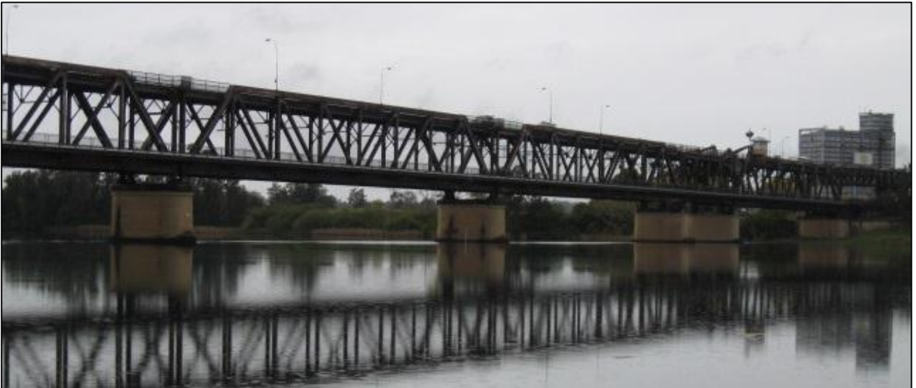
Plate 33: CZB36, north-west facing photograph of Grafton bridge (CZB36) from northern bank of the Clarence (Source: Biosis 2012).
