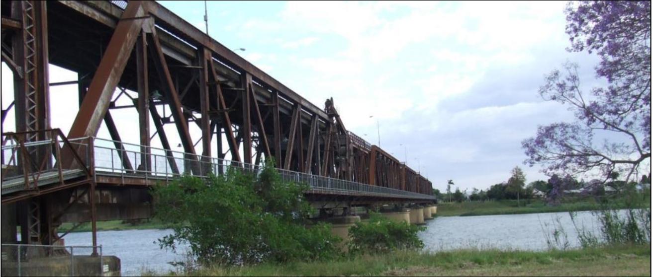
Plate 32: CZB36, north-east facing photograph of Grafton bridge (CZB36) from southern bank of the Clarence (Source: Biosis 2014).
