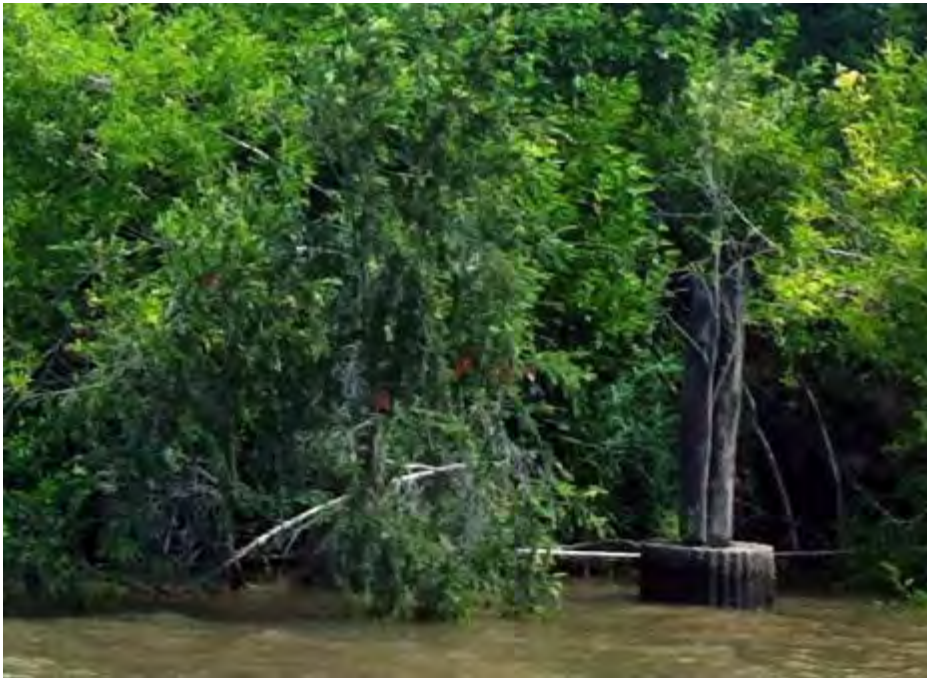
Photograph 15: Exposed remains of timber post with concrete sleeve at base near river bank – showing corrugated outer surface of the sleeve
