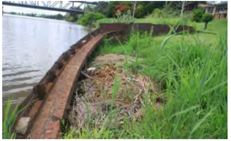
Photograph 24: View east along port quarter to bulk head behind bow with intact topside of hull and reed growth inside hull
