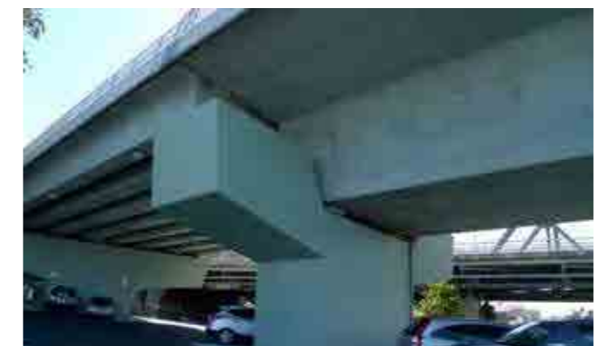
Plate 6.8: Transition pier between box girder and Super T girders at the new Iron Cove Bridge.
