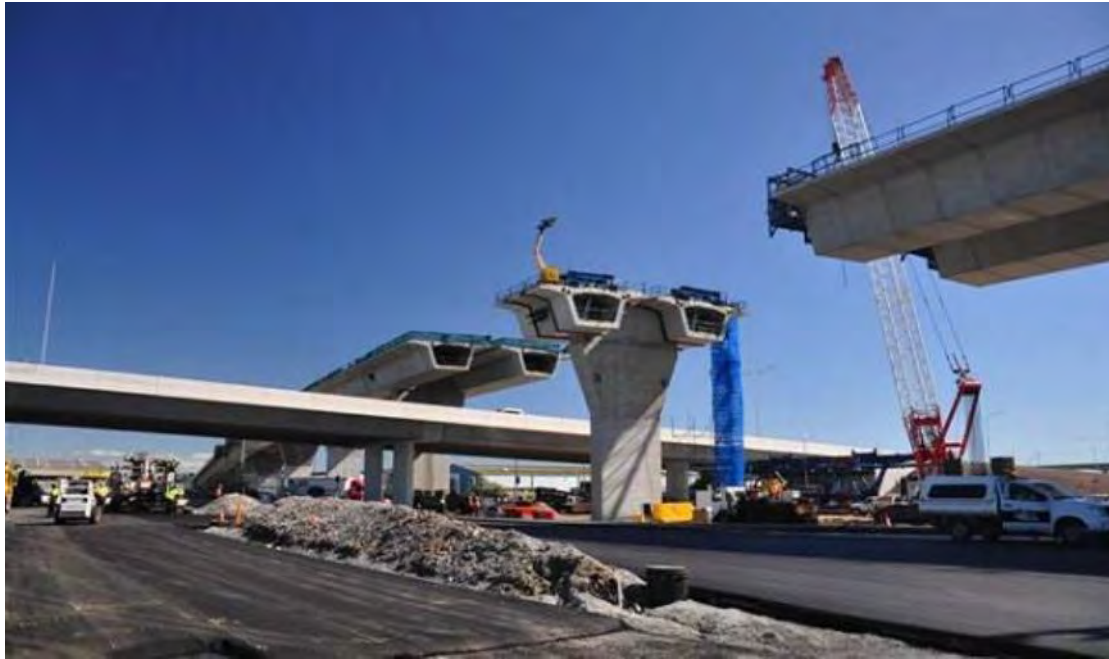
Figure 6-2 Example of balanced precast cantilever construction method – Brisbane Airport Roundabout Upgrade (Source: Arup, 2010)
