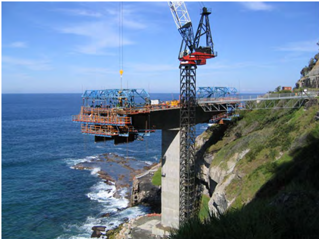
Figure 6-3 Example of insitu balanced cantilever construction method – Sea Cliff Bridge (Source: DLH Alliance, 2004)
