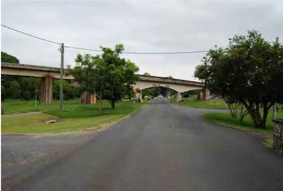
Plate 32: Pound Street Viaduct, listed individually on the LEP, s170 register and the REP.
