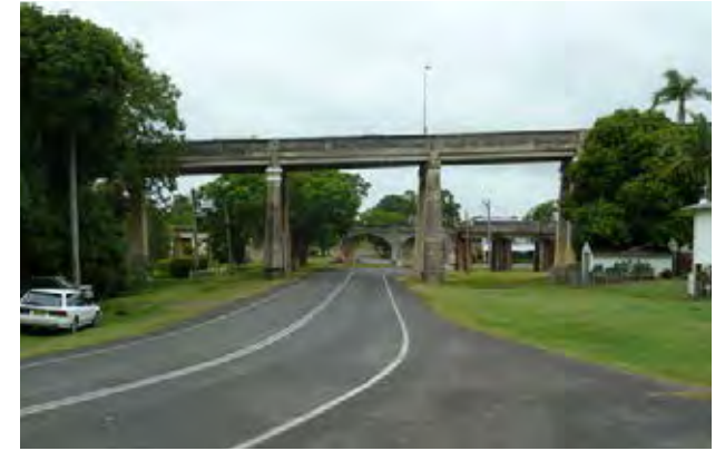
View of the existing viaduct network in Grafton that would be adjacent to Option A
