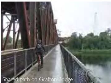
Shared path on Grafton Bridge
