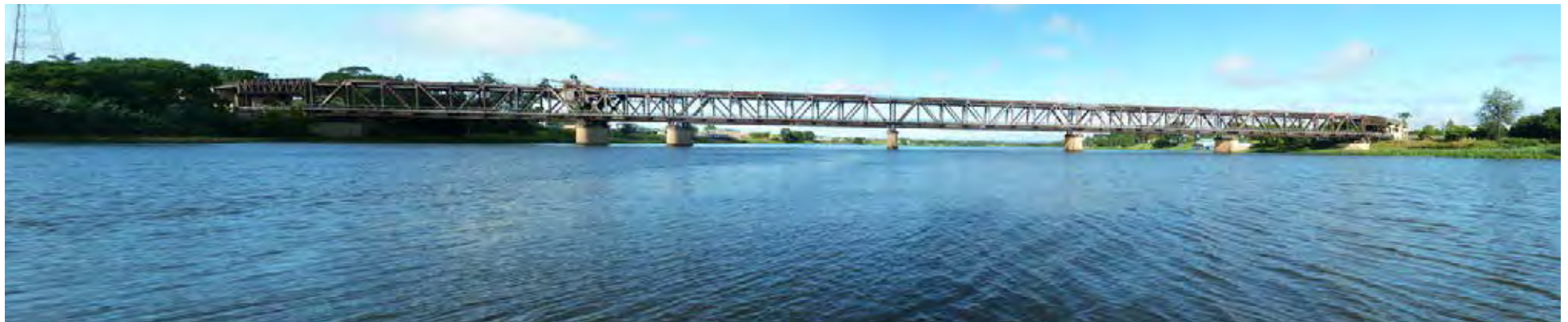
Downstream view of the Grafton Bridge where Option C alignment would cross the Clarence River
