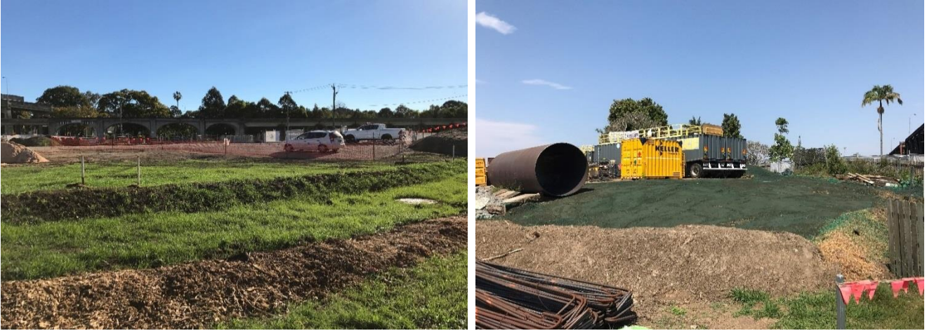
Figure 7 Controls in Grafton (a) mulch bund and seeded earth mounds and; (b) exposed areas banded and polymer applied
