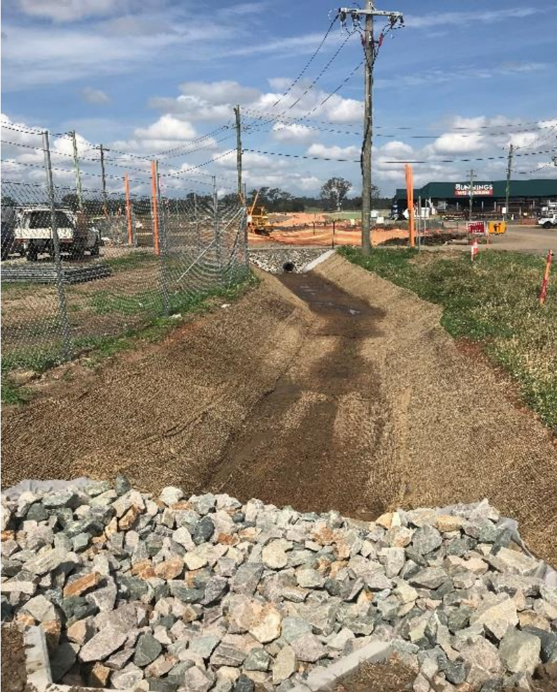
Figure 3 jute mesh lined drains completed to final design at Iolanthe/ Through Street
