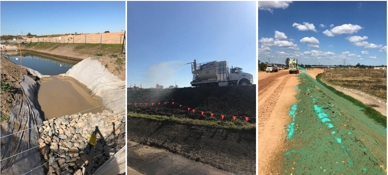
Figure 8 Controls in South Grafton (a) sump removing sediment prior to entering sediment basin; (b) hydroseeding of topsoiled batters and; (c) polymer application on exposed batters
