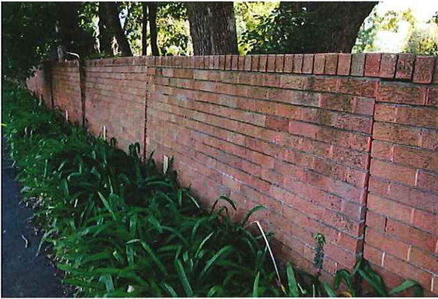
4. The view looking back from the Pacific Highway illustrating the extent of typical movement. The panels are nominally 3000mm long and between 1200mm and 1500mm high.
