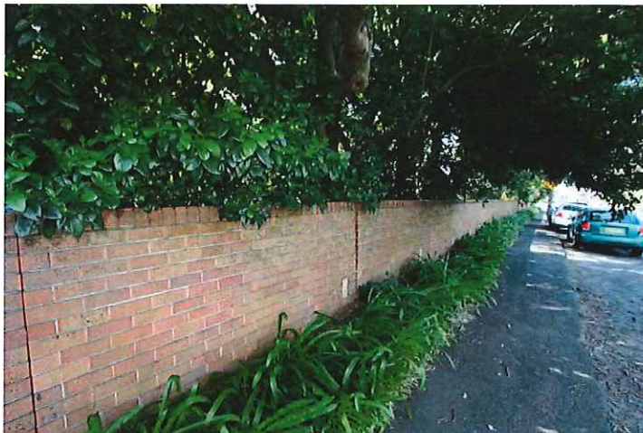
2. View looking down Fox Valley Road to the Pacific Highway. The wall is nominally 1200mm high to this portion of the boundary.
