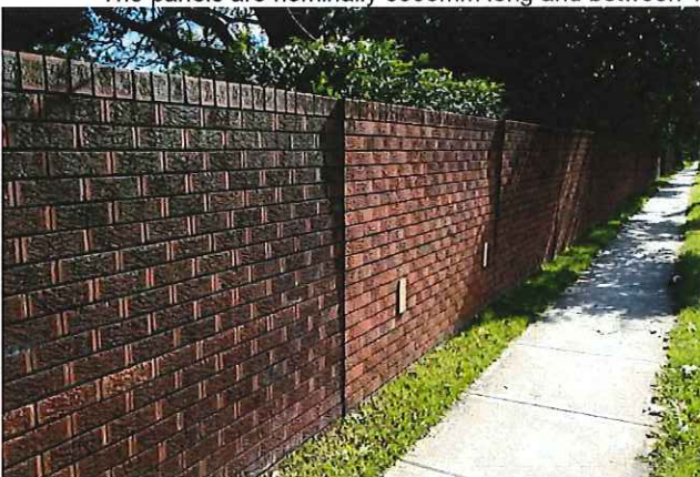
5. A general view looking up the Pacific Highway illustrating the number of panels with movement.
