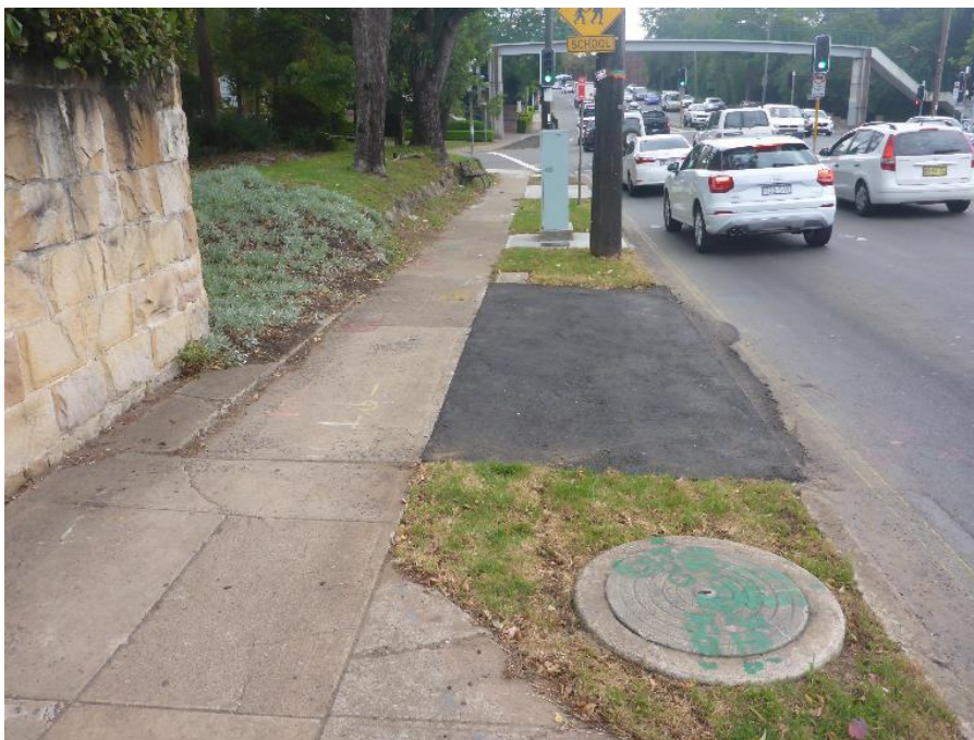
Plate 9 Evidence of sub-surface works within the road reserve in the vicinity of the stone boundary wall of Estha [15], facing north-west
