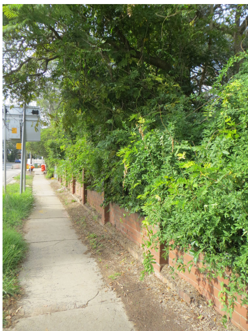
Figure 3-24: Existing brick wall and vegetation at 1482 Pacific Highway, Turramurra (looking east from the Pacific Highway)
