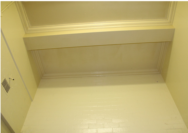
Figure 5.20: Detail of ceiling and brick walls in entry space for booking office (Source: Jacobs 2020)
