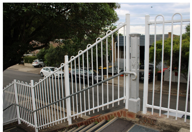
Figure 5.46: Detail of fencing on stairwell leading to Platform 4, facing north (Source: Jacobs 2020)
