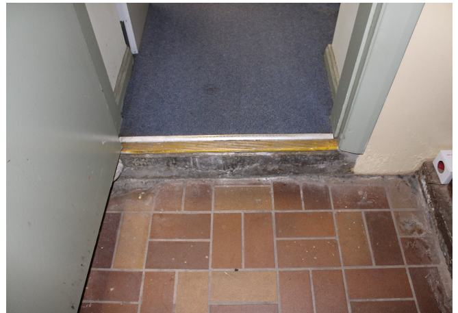
Figure 5.21: Detail of tiling in front of entrance to booking office (Source: Jacobs 2020)
