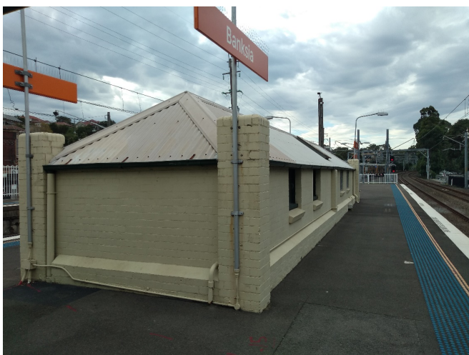
Figure 5.30: Exterior of vaulted roof, located on Platform 2/3, facing north west (Source: Jacobs 2020)
