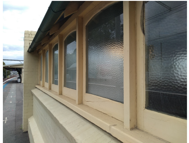
Figure 5.37: Detail of exterior windows of stairwell lantern structure, facing south east (Source: Jacobs 2020)
