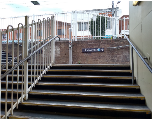
Figure 5.9: Detail of subway entrance on Railway Street side, facing west (Source: Jacobs 2020)
