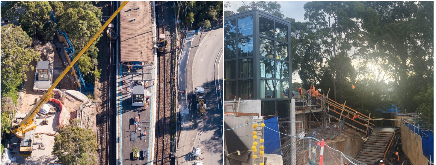
Sneak peak: work progressing on the retaining wall and Como Parade lift.
