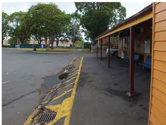
Figure 4.12 Graded asphalt and awning installed in the 1990s, adjacent to the circular driveway.
