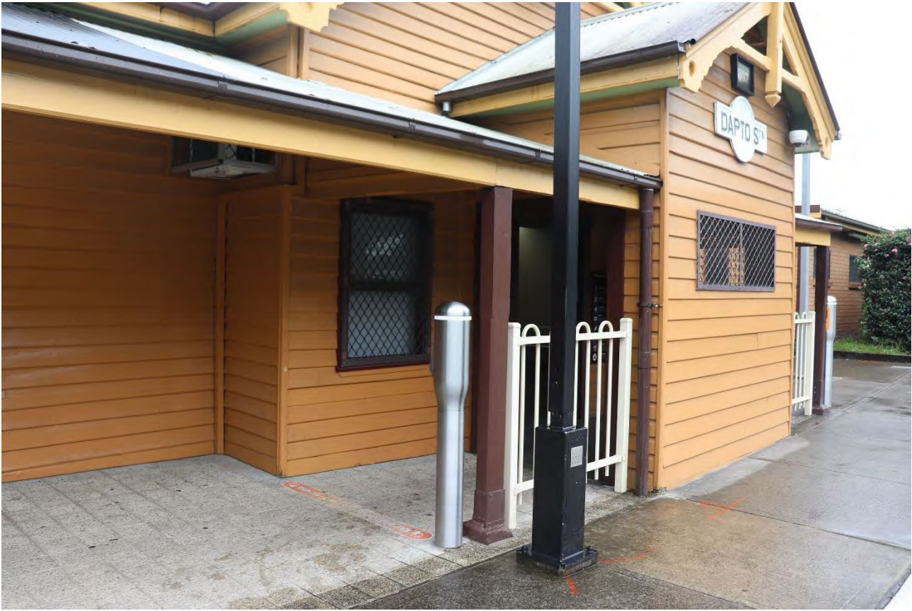
Plate 4.23 Eastern verandah awning showing the former verandah incorporated into building length verandah extension
