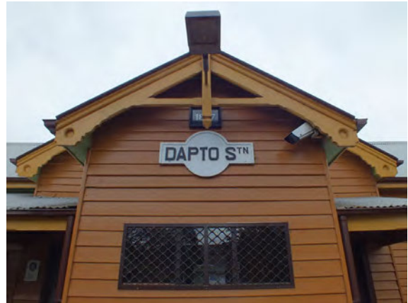
Figure 4.11 Station signs at the entry porch. The original vertical window below the sign has been replaced with a small horizontal window and a CCTV camera attached below the bargeboard.
