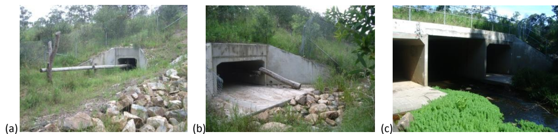
Plate 2: Monitored fauna culverts along the C2HC upgrade at Kew (a), John’s River (b) and Moorland (c).
