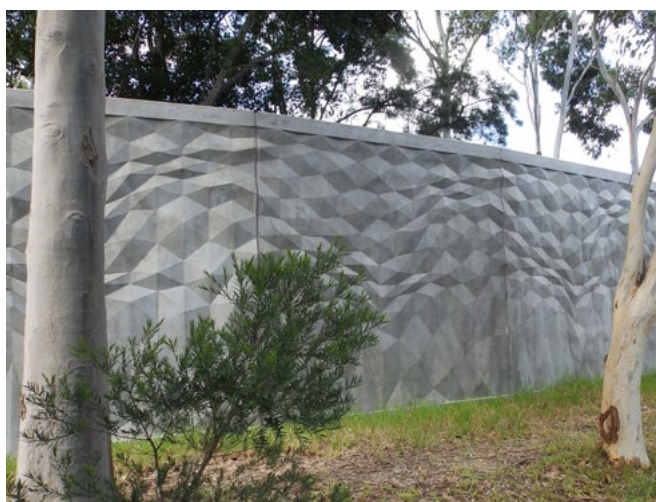
These precast concrete, full height panels at Sexton Place above the Warringah Expressway in Cammeray have a sculptural design on the front face that is both decorative and helps deter graffiti.
