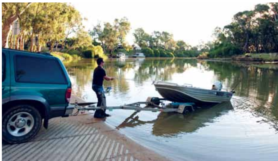
McLeans Beach boat ramp, completed in November 2009 by Deniliquin Shire Council with 50 per cent funding from NSW Maritime's Better Boating Program.
