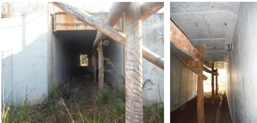
Figure 8. (Left) Entrance to the eastern fauna underpass. (Right) This underpass had a camera installed 2.5 m high to record any animals using the fauna furniture.
